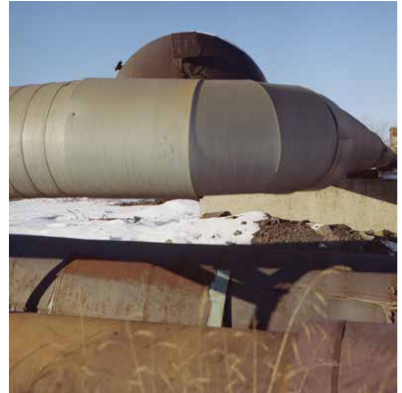
Hot water pipes for the town's heating system. They are above ground because of the permafrost.
